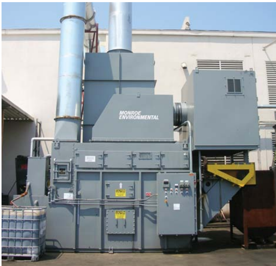
15,000 CFM Dual Throat Venturi Scrubbing System at grease production plant
